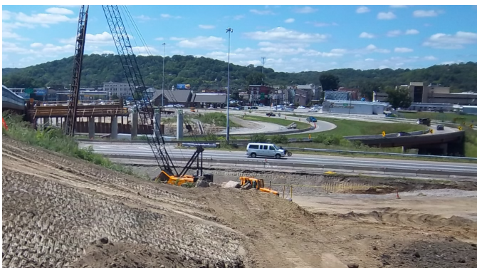
Looking West from Central Parkway, construction proceeds on the new Hopple Street Bridge, which will "flyover" Central Parkway into a straightened MLK Blvd.
