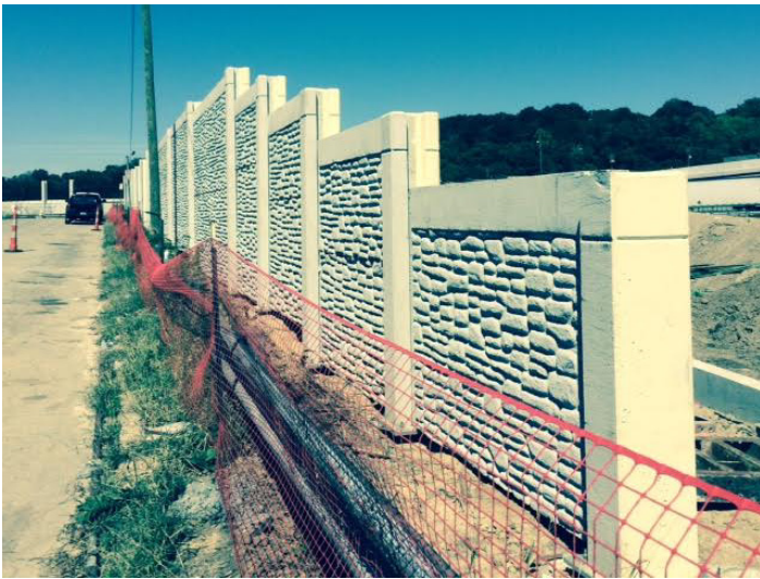
This is Camp Washington's new Noise Wall along Massachusetts (North of Hopple).
